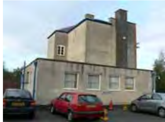
Poor quality extension on School Lane having no respect for the plan form, scale or original design features along with poor fenestration pattern, materials and roof
