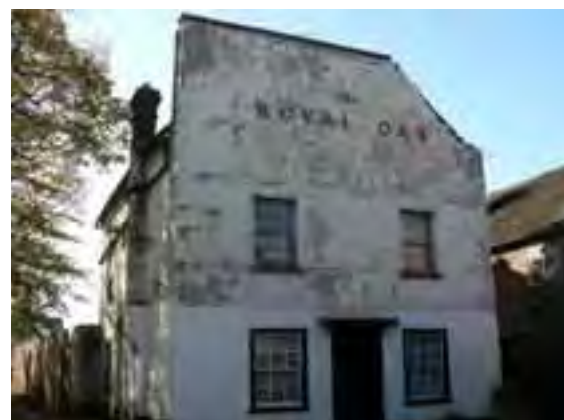
Royal Oak building in Court Row in disrepair
