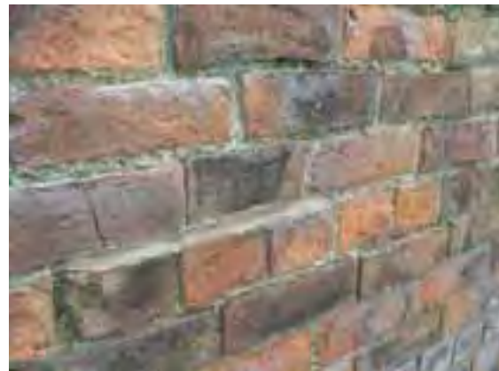
Unsympathetic repointing on Waterside
