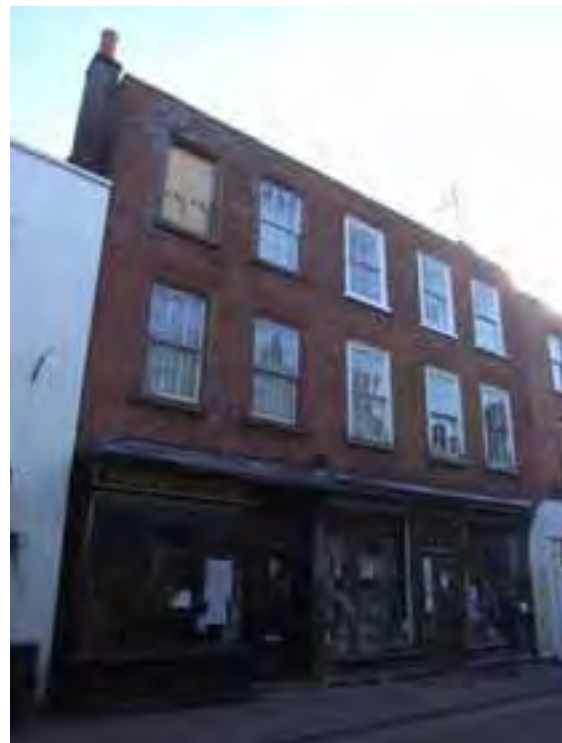
Boarded up windows above shop on Old Street
