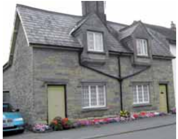
And again in The Village. Note slate roof on this C19 building
