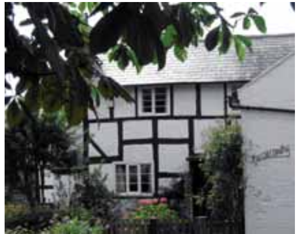
Typical window pattern – following the spirit of an early metal casement. Note changes to framing suggesting a raised roof
