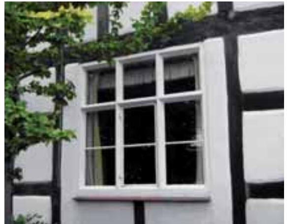
...And another metal window in a changed opening...
