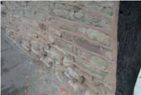
Cement mortar exacerbating weathering of soft local stone
