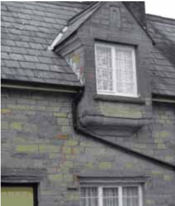
Nineteenth Century traditional dormer translated in stone. Note the stone mouldings and hoods over window and door.
