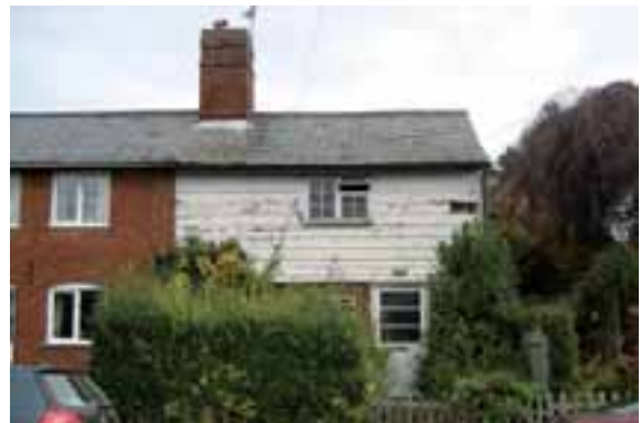
Inappropriate boarding and window design
